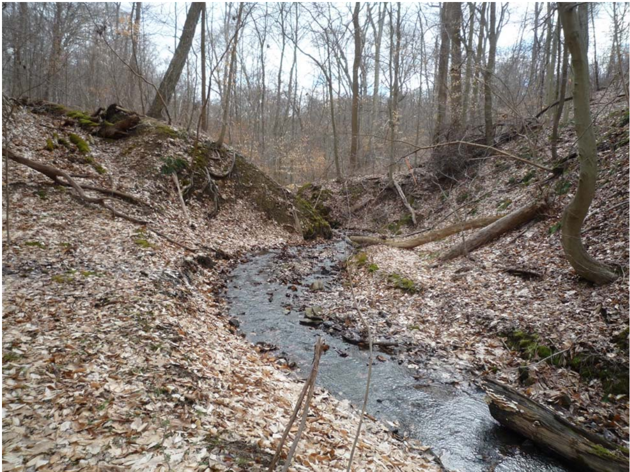
Figure 11. View upstream (west) at the stream eroding the toe of the slide mass on the left, with a tree bent from creep and sliding on the right.
