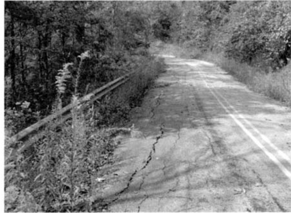
Figure 16. View of Landslide 6 looking east.
