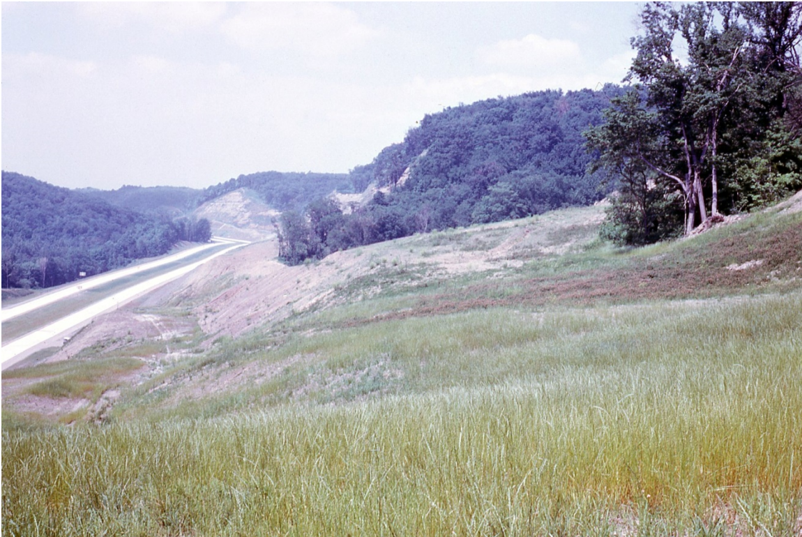
View north from approximate Sta 895 at the excavated slide debris above the lower excavated bench on top of the Saltsburg shale and sandstone.
