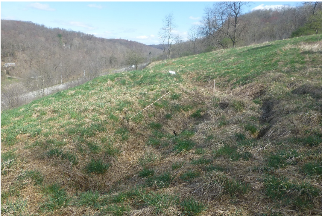
View north at the above-mentioned cracks. Clipboard and 6 foot rule for scale.
