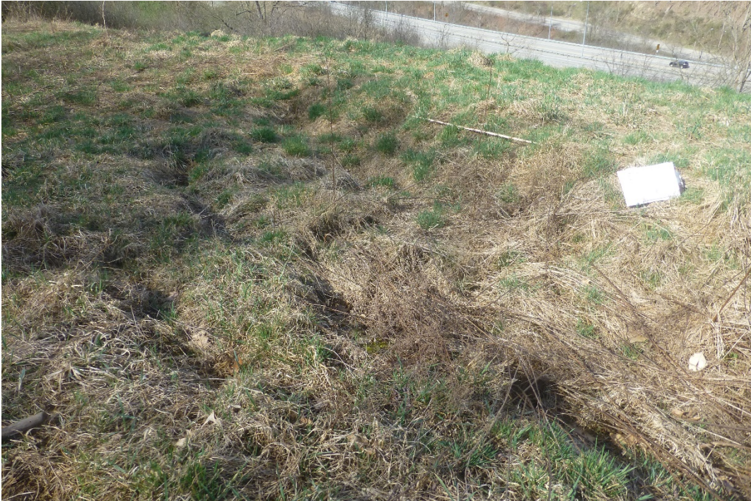
View southwest at the cracks in the slide debris. Clipboard and 6 foot rule for scale. Approximate Sta 904.
