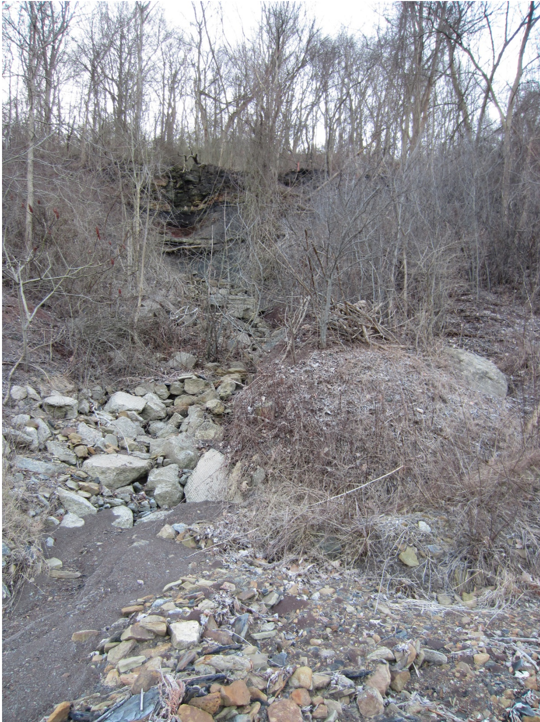
Overall view northeast at the eroded ravine Sta 976.
