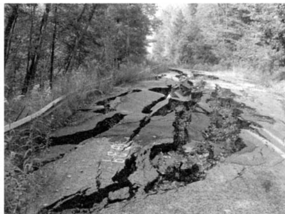
Figure 14. View of Landslide No. 4 looking east.
