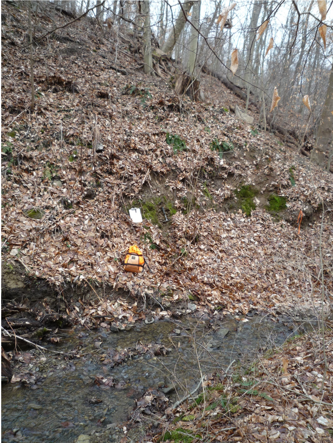
Overall view of slumped Pittsburgh red beds shaly claystone on the slope on the north side of the stream at approximate el. 980 ft.
