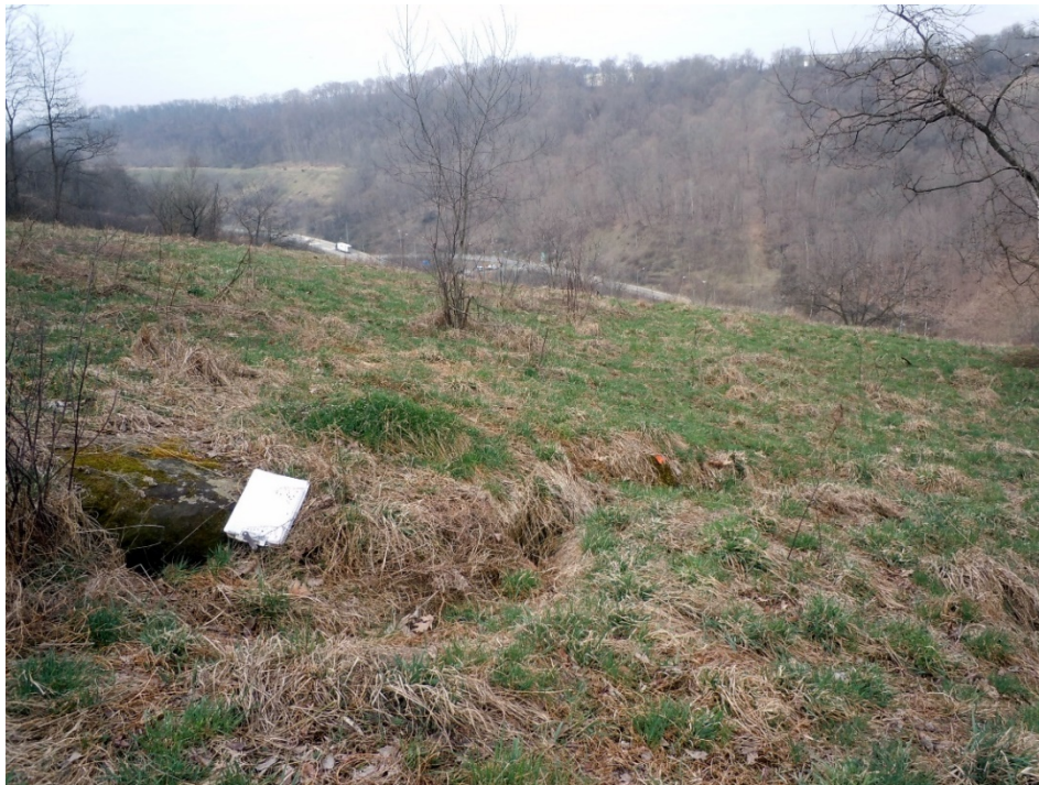
View southwest at the cracks between sandstone slide blocks. Clipboard for scale. Approximate Sta 907.
