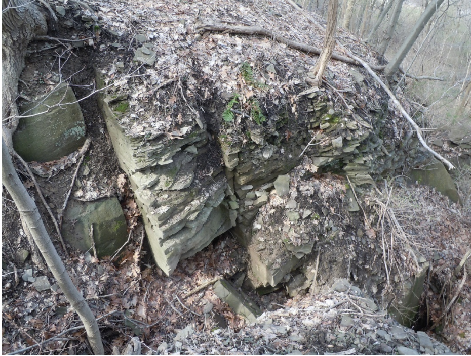
View south at the slide fissure at approximate Sta 906.
