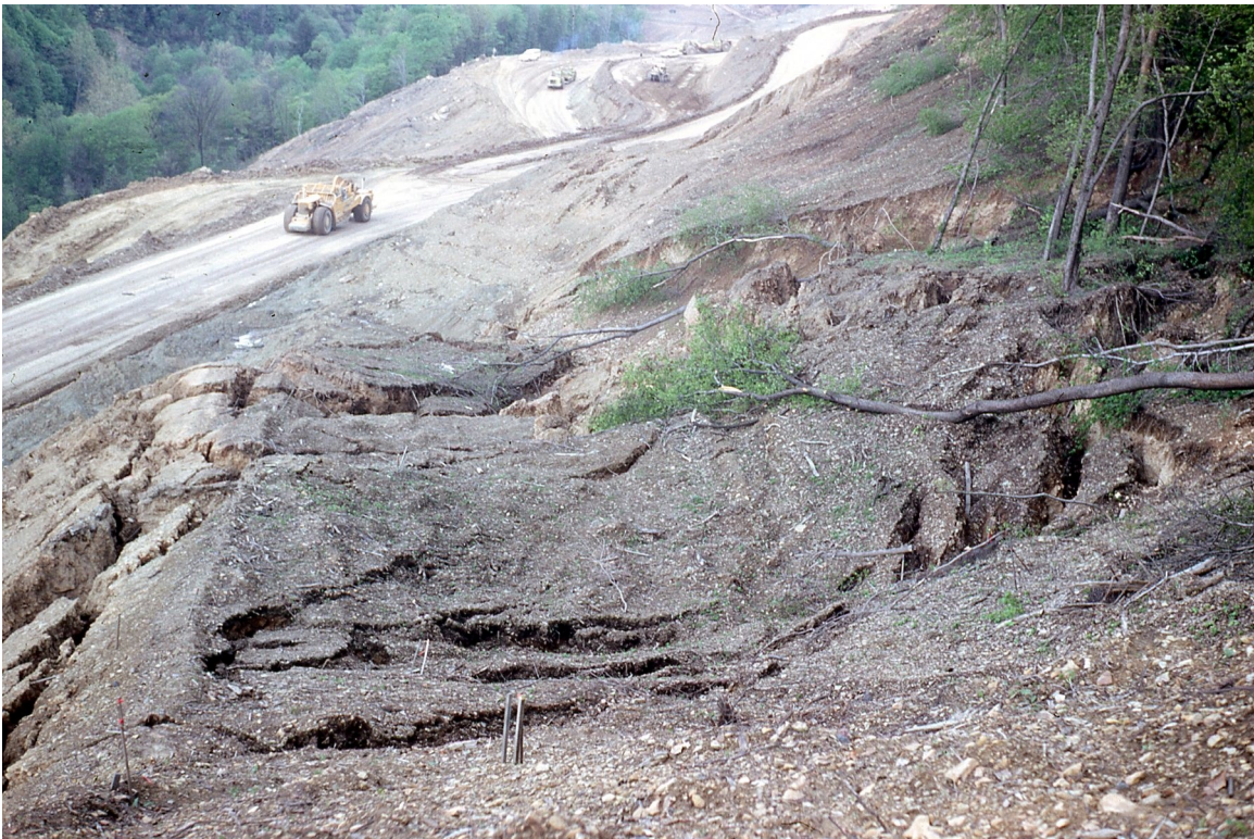
I-79 Station 916-918 Progressive Failure of Colluvial Slope – March 13, 1969
