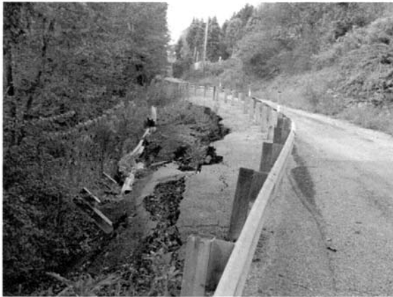
Figure 11. View of Landslide No. 1 looking west.
