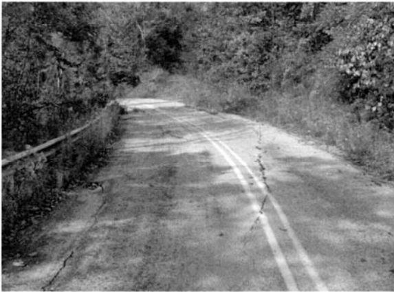
Figure 15. View of Landslide 5 looking east.
