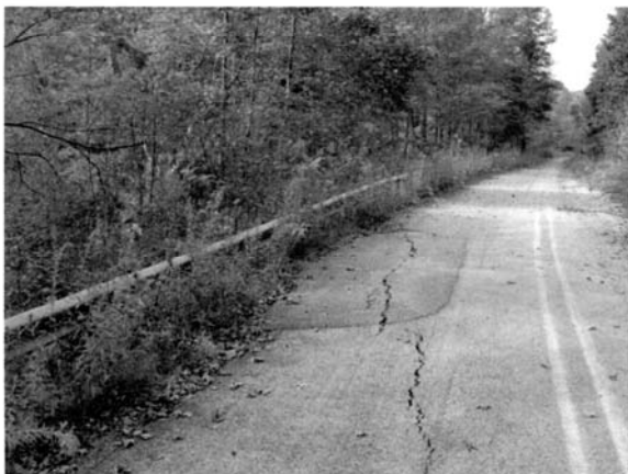
Figure 13. View of Landslide No. 3 looking east.
