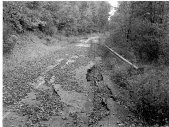
Figure 12. View of Landslide No. 2 looking east.
