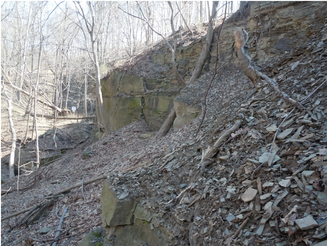
View north along the slide scarp from approximate Sta 904. The graben is at the top left.
