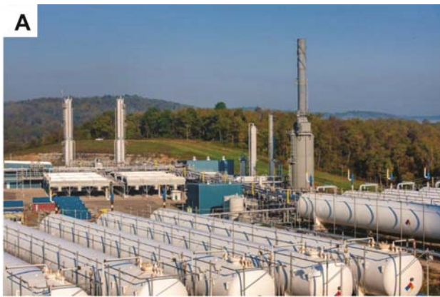
Figure 55. Photographs of the MarkWest Houston Complex in Houston, PA. A, the MarkWest Houston Plant extracts and separates higher hydrocarbons from the “wet” Marcellus shale gas produced in this area. Source: MPLX Image Gallery ( http://www.mplx.com/content/inline-images/mpc/about/image_gallery/markwest/7028za_2172m.jpg ). B, the MarkWest Houston Plant has a large control room manned 24 hours a day. Source: MPLX Image Gallery ( http://www.mplx.com/content/inline-images/mpc/about/image_gallery/markwest/7028za_5009m.jpg ).
