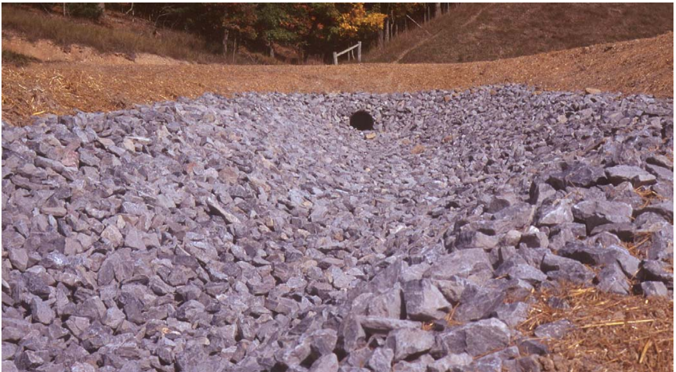
Figure 34. Spillway at Brushy Fork dam after repair, approximately one year later. Photograph was taken in the same direction as in Figure 33 but from about 50 feet east up the spillway. All Foreknobs strata have been covered by ballast.
