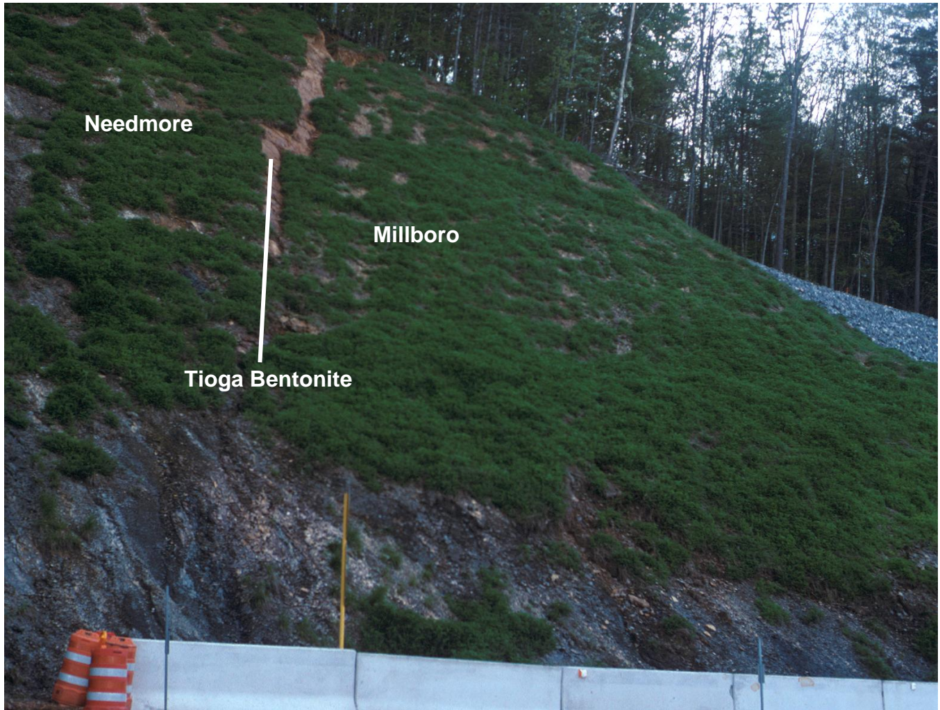
Figure 12. Landslide initiated in the Tioga Bentonite, US 250, east of Monterey, VA. Strata of the Millboro Shale are sliding downhill along a waterlogged Tioga Bentonite. Concrete barriers have been erected to keep slide material off the highway. Ballast on the right covers an earlier Millboro slide scar.
