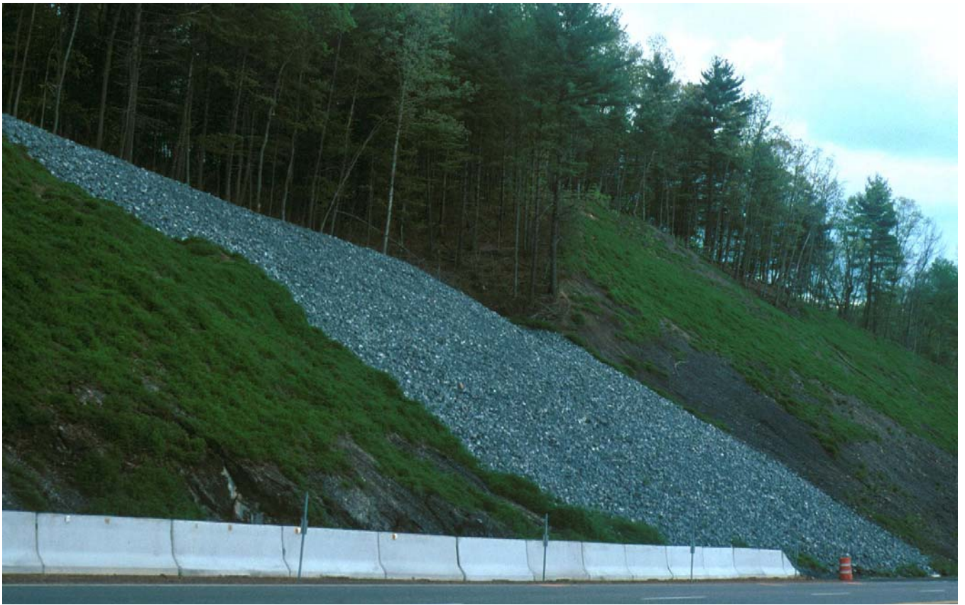
Figure 13. Rock ballast covers an earlier landslide surface in the Millboro Shale, US 250, east of Monterey, VA.
