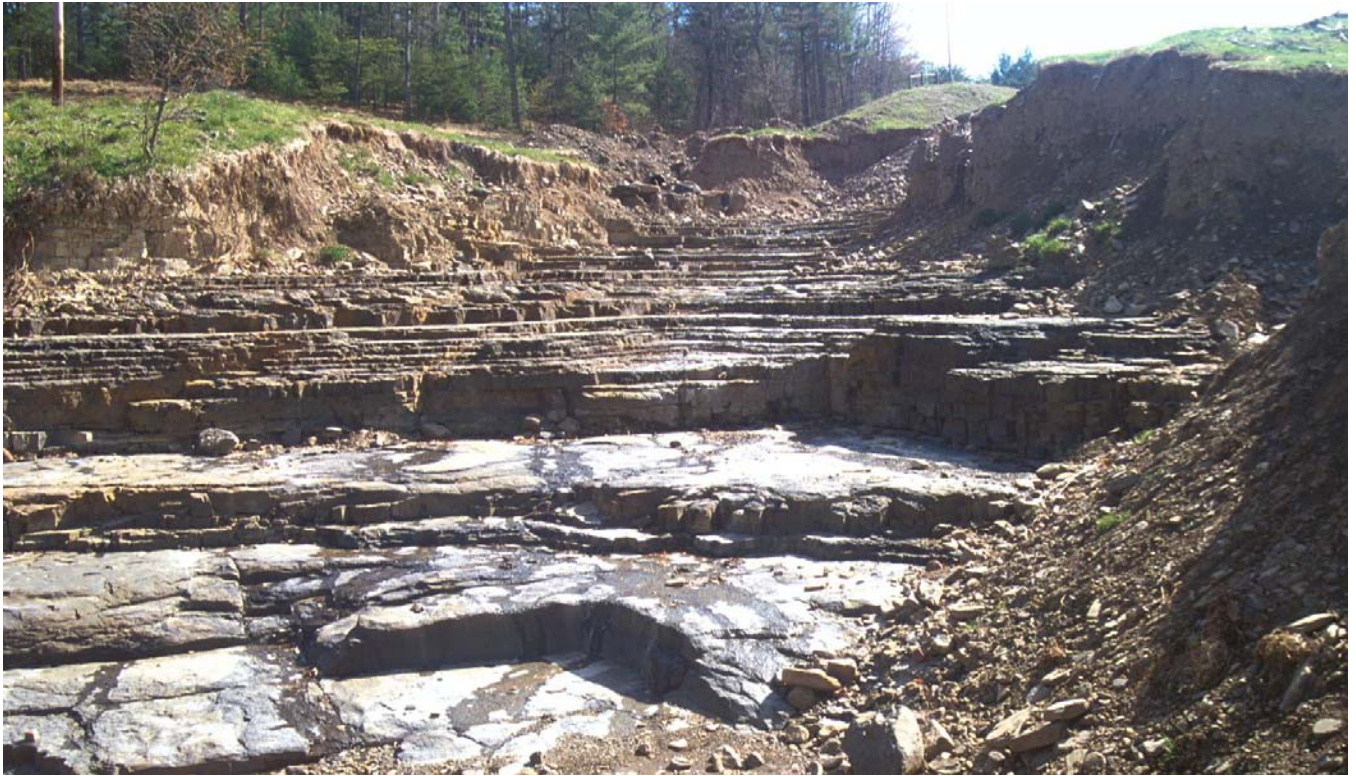
Figure 33. Eroded spillway following heavy rains from Hurricane Fran (Sept. 1996) and overtopping of Brushy Fork soil conservation dam just to the south. The exposed rock unit in the foreground is the Devonian Foreknobs Formation.
