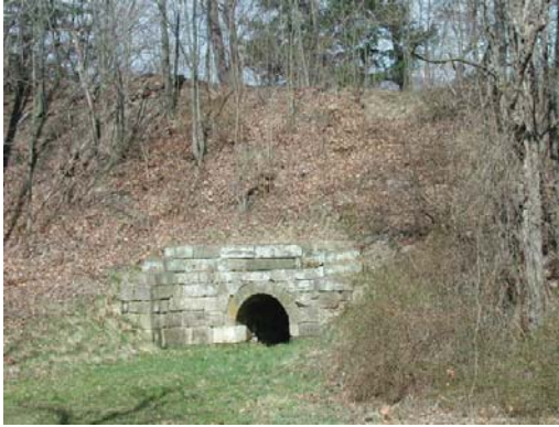
Figure 28. Photograph of the culvert beneath Inclined Plane No. 10 near Foot of Ten.
