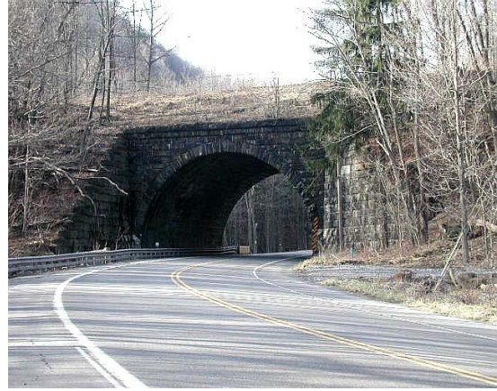
Figure 32. Photograph of the Muleshoe Curve Bridge, formerly used by the New Portage Railroad and the Pennsylvania Railroad.
