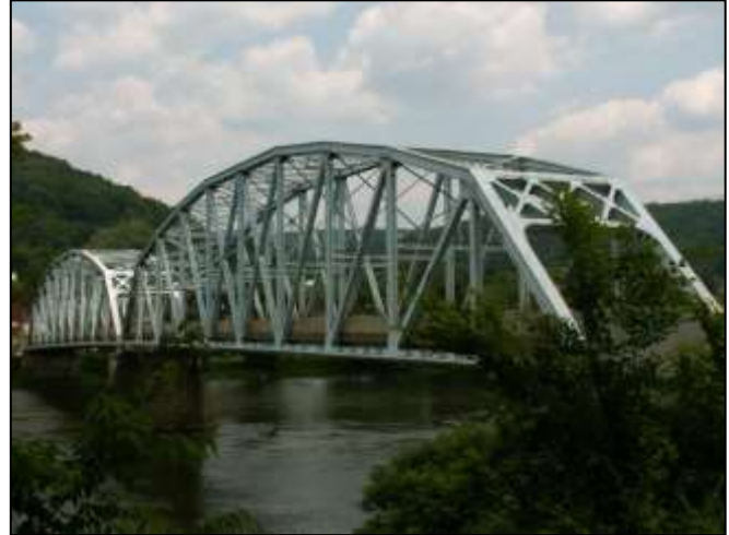
Tidioute Bridge, site of the annual reenactment of The Bridge at Remagen
