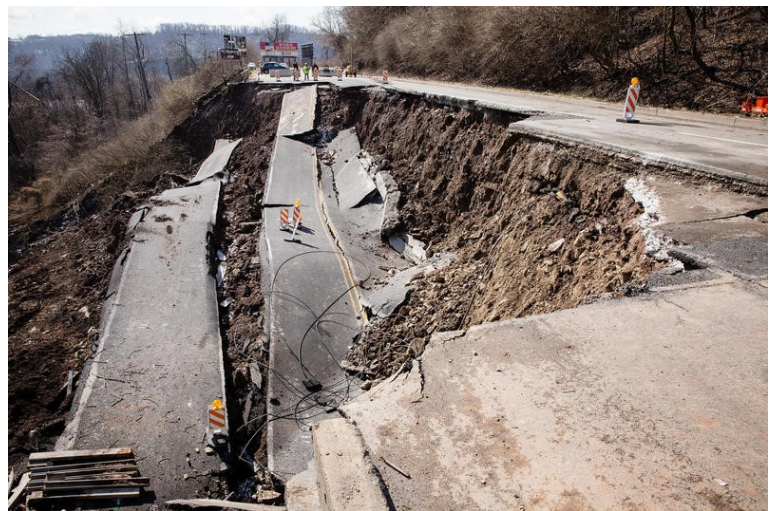
Students need to be trained less about finding resources and more about assessing the potential for, and mitigating, things like the damage from a landslide that occurred on Route 30 in East Pittsburgh in 2018.
