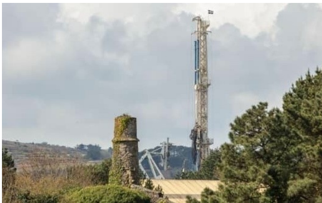
Photograph of a rig drilling a deep geothermal well in Cornwall, England.
