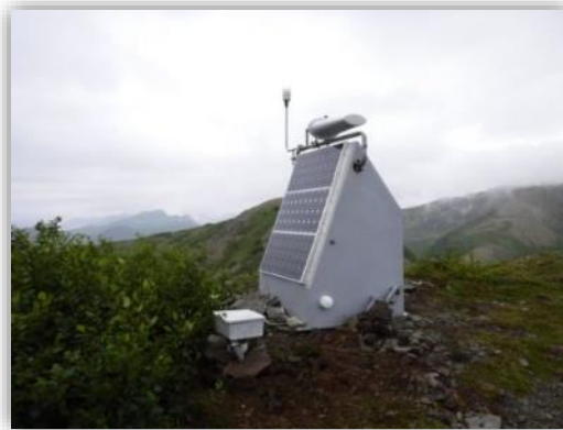
ESTA station P19K, one of the stations closest to the Iniskin earthquake of 2016. Solar panels power the station, and the seismometer is buried in a borehole to insulate it from surface noise.
